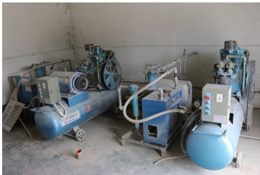
Figure 45. Pneumatic system (Air-compressor equipment)
