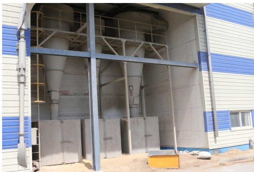
Figure 46. Dust collector (Cyclones)
